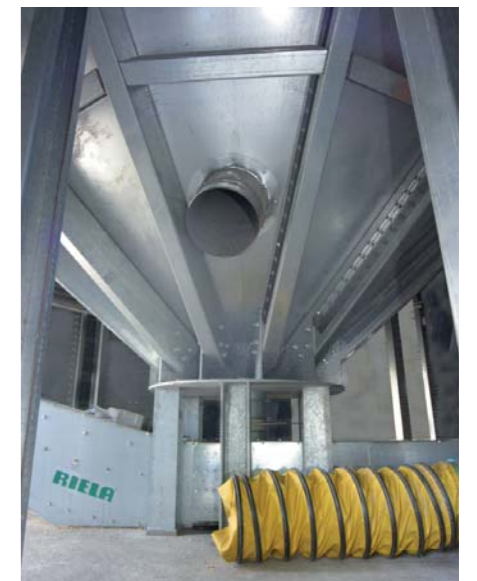
Silo funnel with ventilation connection
