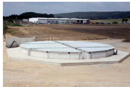
Ventilation ducts in the silo base
