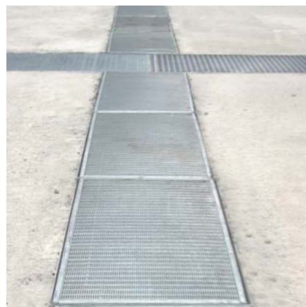
Grids on ventilation ducts
